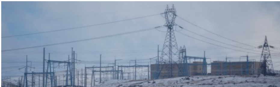
Celilo Station, the northern terminus of the Pacific DC Intertie. | © RTO Insider
